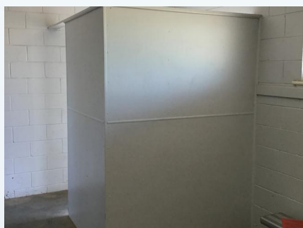
PHOTO NO.: J163425-9235A-PHOTO031 RESULT: ASBESTOS - POSITIVE BUILDING/LEVEL: CHANGE ROOMS - GROUND LEVEL ROOM/LOCATION: FEMALE CHANGEROOM - ADJACENT ENTRY DOOR FEATURE/MATERIAL: PARTITION WALL - FIBRE CEMENT SHEETING SAMPLE NO.: J163425-9235A-015
