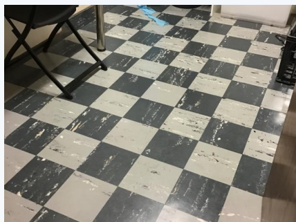
PHOTO NO.: J163425-9235A-PHOTO045 RESULT: ASBESTOS - POSITIVE BUILDING/LEVEL: CHAPEL, BISHOP GALLAGHER, CANTEEN & STAFF BUILDING - GROUND LEVEL ROOM/LOCATION: MAKEUP / STORE ROOM - THROUGHOUT FEATURE/MATERIAL: FLOOR COVERING - VINYL TILES & ADHESIVE SAMPLE NO.: J163425-9235A-023
