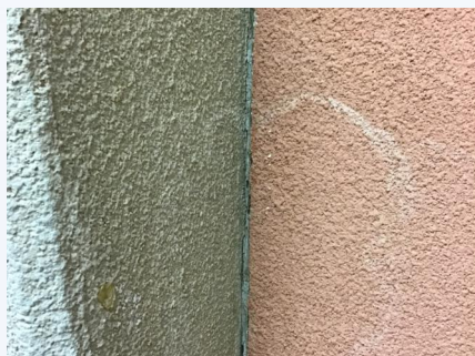
PHOTO NO.: J163425-9235A-PHOTO047 RESULT: ASBESTOS - POSITIVE BUILDING/LEVEL: CHAPEL, BISHOP GALLAGHER, CANTEEN & STAFF BUILDING - GROUND LEVEL ROOM/LOCATION: - VARIOUS THROUGHOUT FEATURE/MATERIAL: EXPANSION JOINT - CONSTRUCTION JOINT MASTIC SAMPLE NO.: J163425-9235A-025
