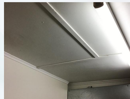
PHOTO NO.: J163425-9235A-PHOTO046 RESULT: ASBESTOS - POSITIVE BUILDING/LEVEL: CHAPEL, BISHOP GALLAGHER, CANTEEN & STAFF BUILDING - GROUND LEVEL ROOM/LOCATION: MAKEUP / STORE ROOM - WEST ROOM FEATURE/MATERIAL: CEILING LINING - FIBRE CEMENT SHEETING SAMPLE NO.: J163425-9235A-024
