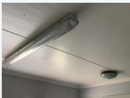
PHOTO NO.: J163425-9235A-PHOTO025 RESULT: ASBESTOS - POSITIVE BUILDING/LEVEL: CHANGE ROOMS - GROUND LEVEL ROOM/LOCATION: MALE CHANGEROOM - TOILET FEATURE/MATERIAL: CEILING LINING - FIBRE CEMENT SHEETING SAMPLE NO.: J163425-9235A-013
