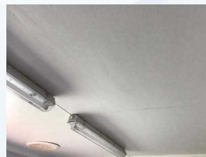
PHOTO NO.: J163425-9235A-PHOTO030 RESULT: ASBESTOS - PRESUMED POSITIVE BUILDING/LEVEL: CHANGE ROOMS - GROUND LEVEL ROOM/LOCATION: FEMALE CHANGEROOM - SHOWERS FEATURE/MATERIAL: CEILING LINING - FIBRE CEMENT SHEETING SAMPLE NO.: SIMILAR TO: J163425-9235A-013
