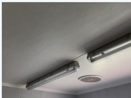
PHOTO NO.: J163425-9235A-PHOTO027 RESULT: ASBESTOS - PRESUMED POSITIVE BUILDING/LEVEL: CHANGE ROOMS - GROUND LEVEL ROOM/LOCATION: MALE CHANGEROOM - SHOWERS FEATURE/MATERIAL: CEILING LINING - FIBRE CEMENT SHEETING SAMPLE NO.: SIMILAR TO: J163425-9235A-013
