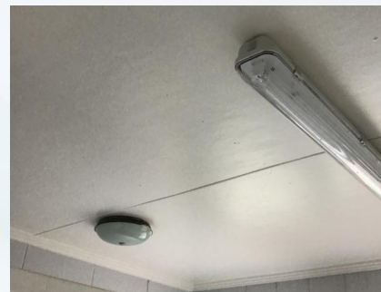
PHOTO NO.: J163425-9235A-PHOTO028 RESULT: ASBESTOS - PRESUMED POSITIVE BUILDING/LEVEL: CHANGE ROOMS - GROUND LEVEL ROOM/LOCATION: FEMALE CHANGEROOM - TOILET FEATURE/MATERIAL: CEILING LINING - FIBRE CEMENT SHEETING SAMPLE NO.: SIMILAR TO: J163425-9235A-013
