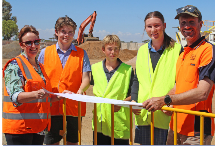
DEVELOPMENT: Work began on the new Boarding House, our current Boarders keen to see each step of the process.
